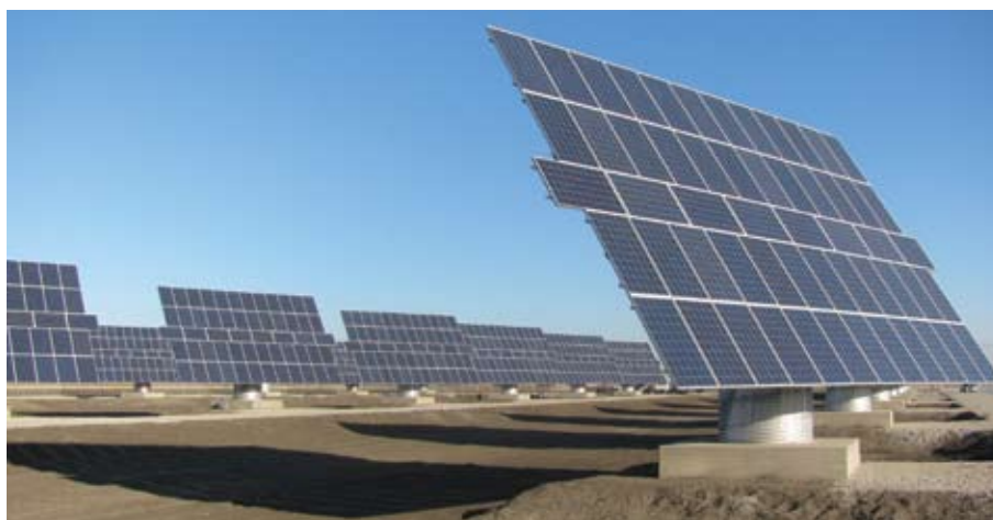
PROINSO is supplying Mecasolar trackers for this 1 MW PV project in California's Madera Water District. Photo courtesy of PROINSO.
